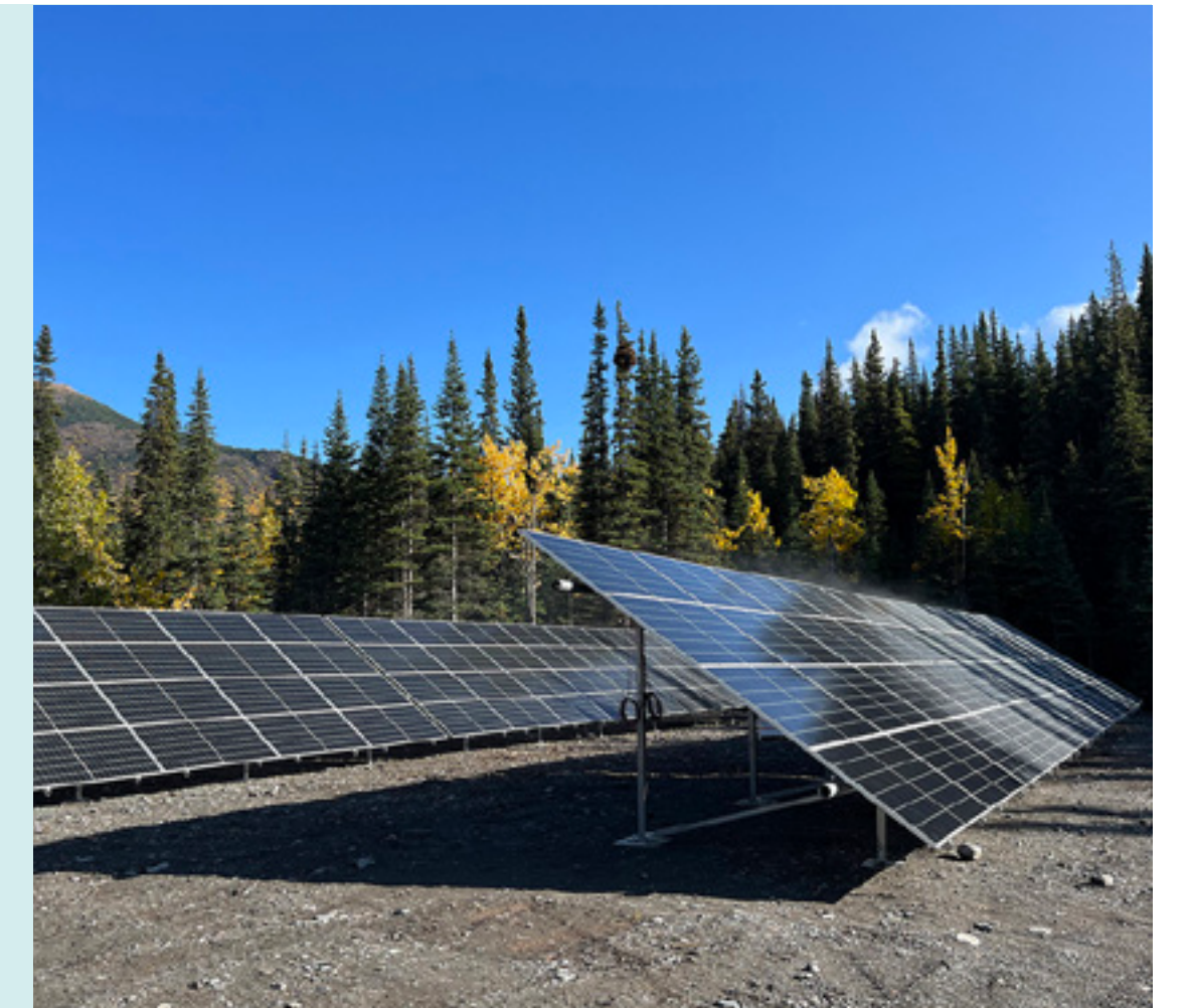
Pictured: Solar Panels at Schaft Creek Development Project.
